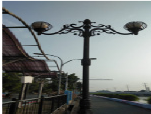
Park Light Not Working
